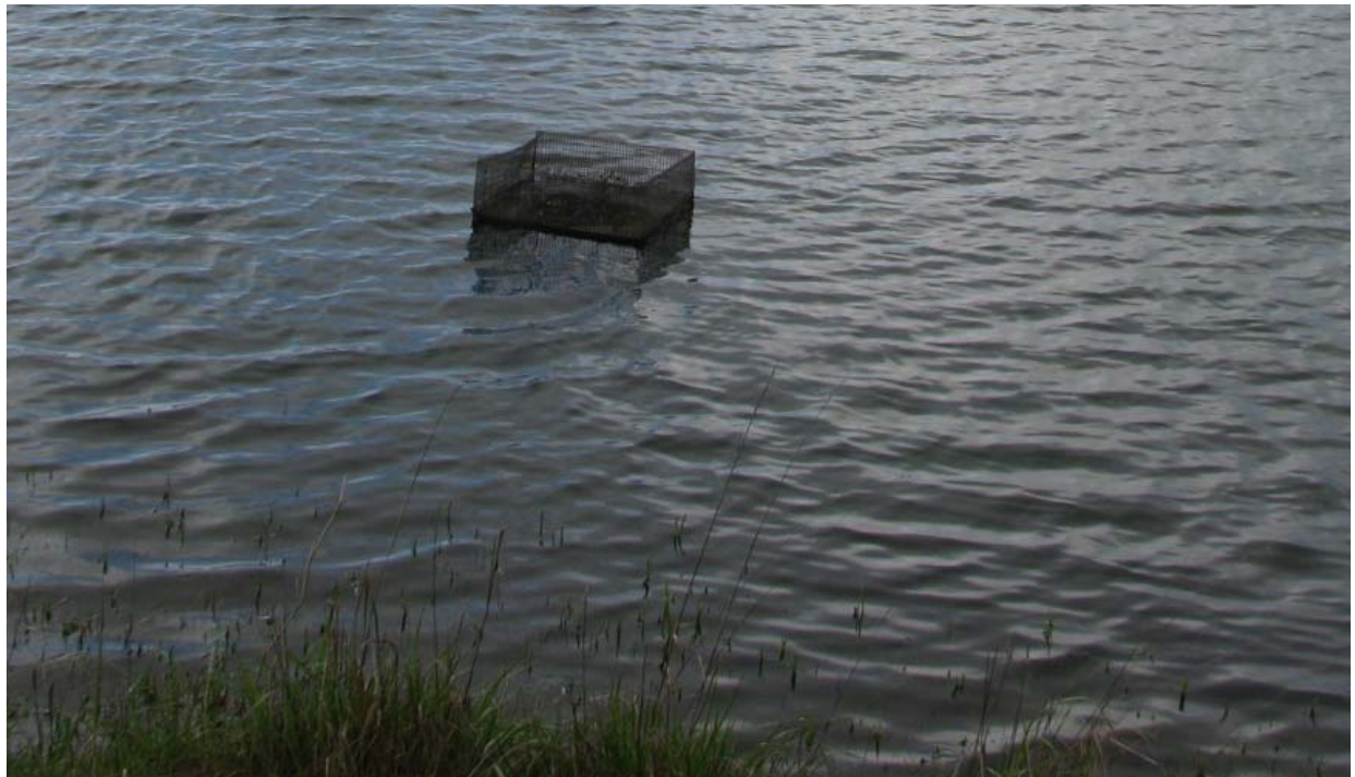
Figure 4. Trickle tube for outlet. The trash rack and general condition appear to be in fair to good condition and it was functioning the day of inspection.
