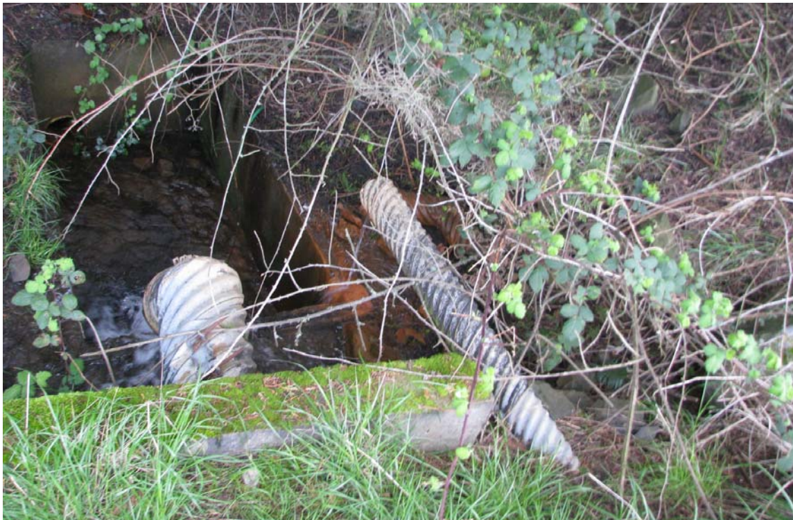
Figure 2. Outlet and toe drain that have some deterioration but are still in fair functional condition. The outlet conduit is not encased and may need to be lined in the next 10-20 years.
