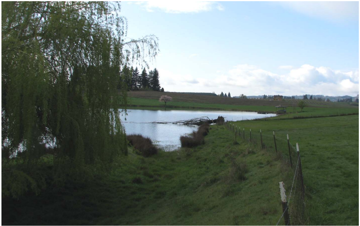
Figure 3. Entrance to the auxiliary spillway. From the lack of erosion and signs of water flow it is rare that water gets into this spillway.
