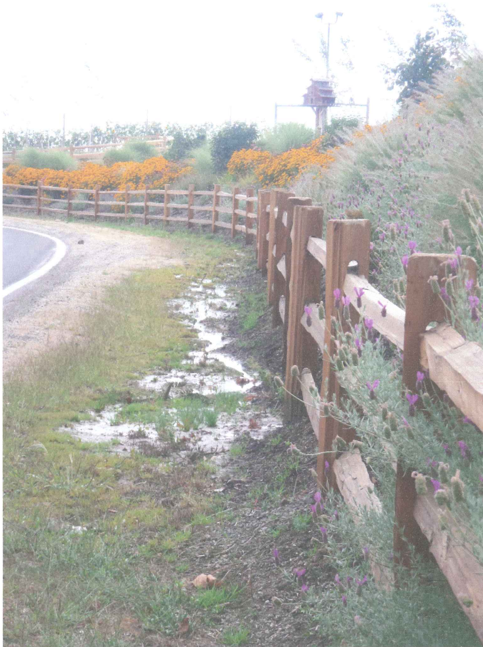
Water in drainage not from rainfall (there was only a trace of rain in the past 24 hrs)
