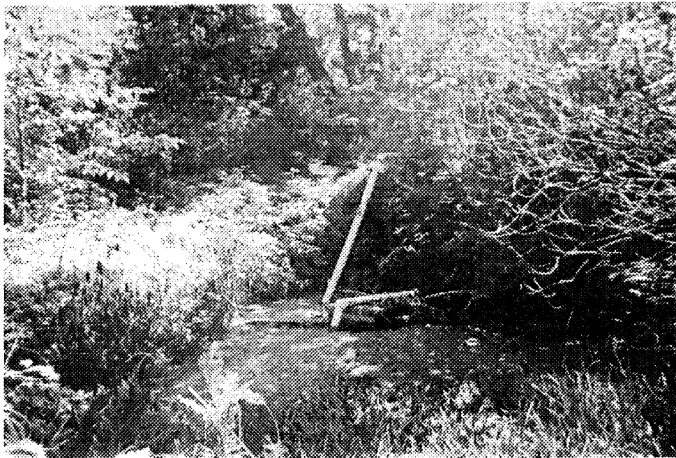
Picture 4. Unit 62 looking upstream. Sandbags form isolated pool on west side of channel for pump house.
