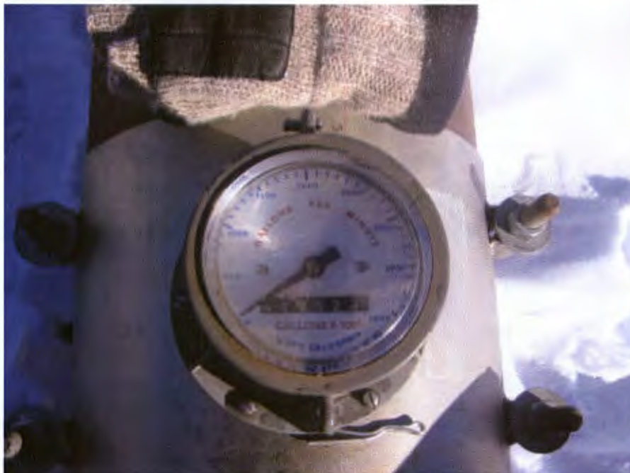
FLOW METER - WELL #1
