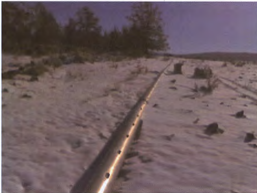
MAIN LINE USED FOR FLOOD IRRIGATION
