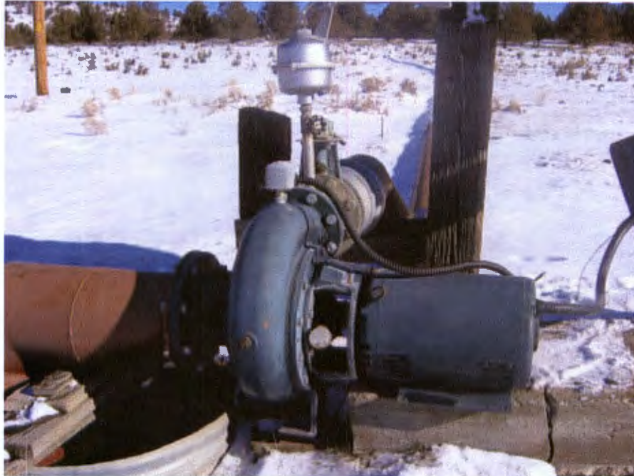
IRRIGATION PUMP AT CANAL, USED FOR FLOODING
