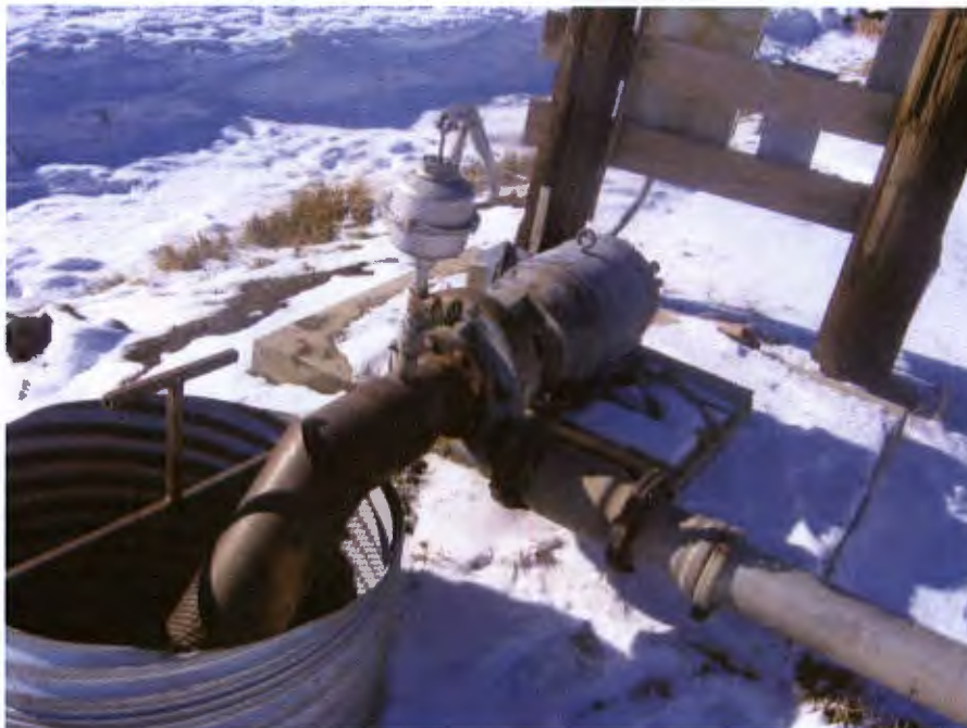
IRRIGATION PUMP AT CANAL, USED FOR PIVOT
