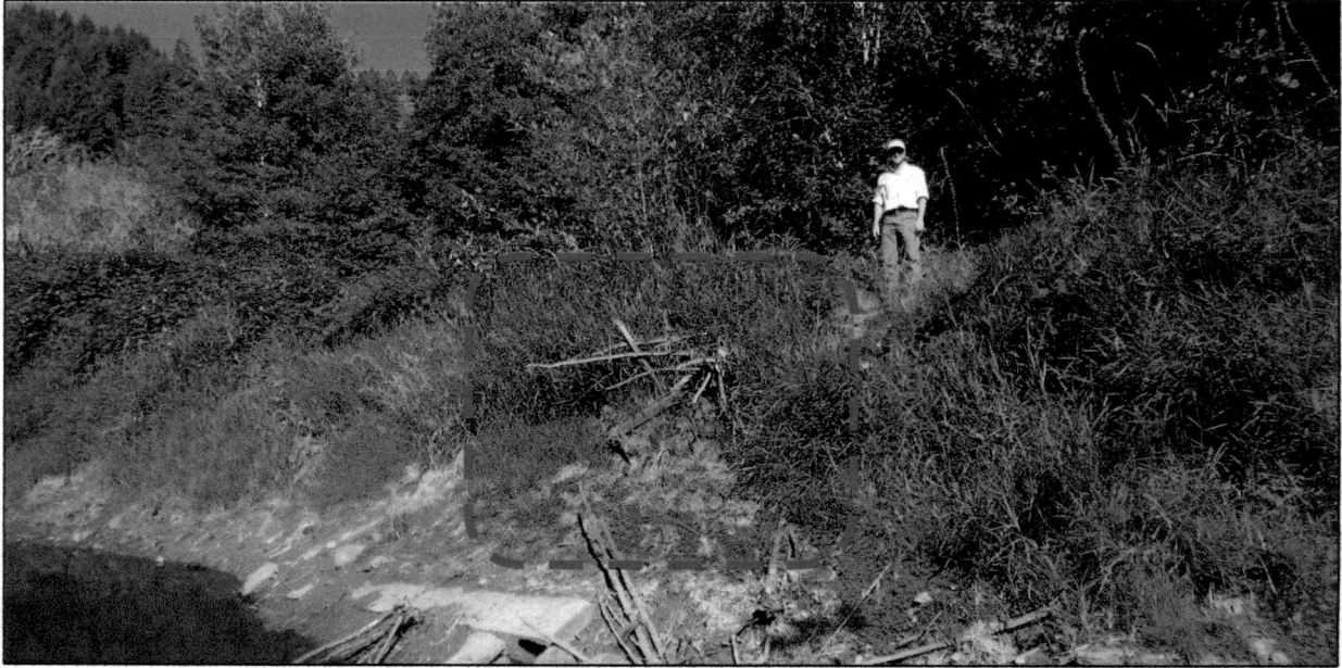
Figure 4-2. The spillway location between the pond and Five Rivers at the southeast corner of the pond. The proposed drop spillway is intended to reduce the effects of debris and provides additional flow capacity through the pipe spillway.
