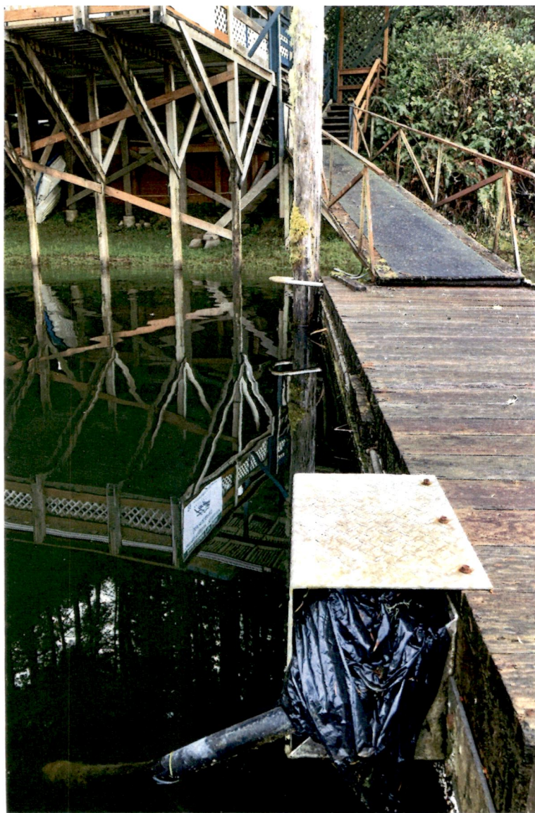
Pump on the Dock.
