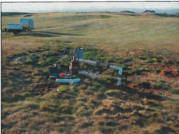
Irrigation Well COOS52219. Note flow meter.
