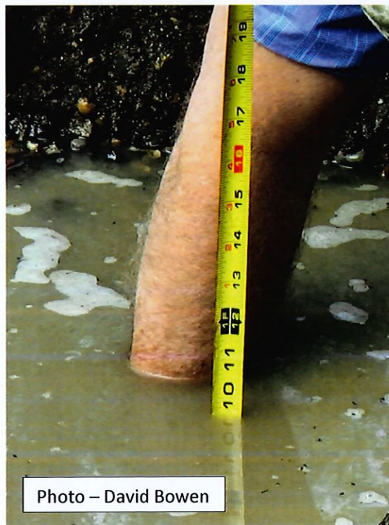
Figure 2. "The water table is lower than the ground level. The tape measure is to the top of the perforated pipe. The water level is about 4-6 inches above the water level. So we have approx. 16 in of cover over the pipe. In probing the ground trying to find the pipe. It appears to hit bedrock at approx. 28 inches +/-." – David Bowen; Email 10/28/2020.
