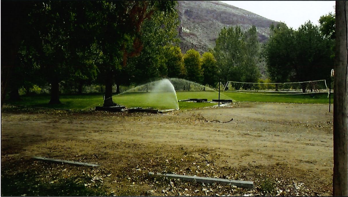
Figure 5: Sprinklers operating during flow measurement.
