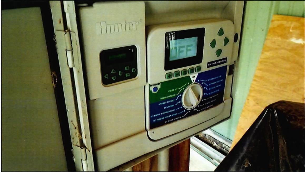
Figure 3: Irrigation system controller.
