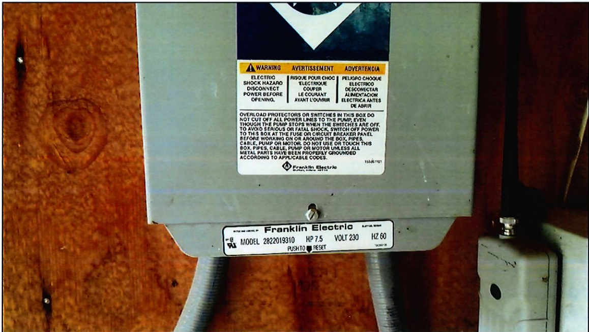
Figure 4: Franklin Electric motor control box indicating pump may be 7.5 hp.
