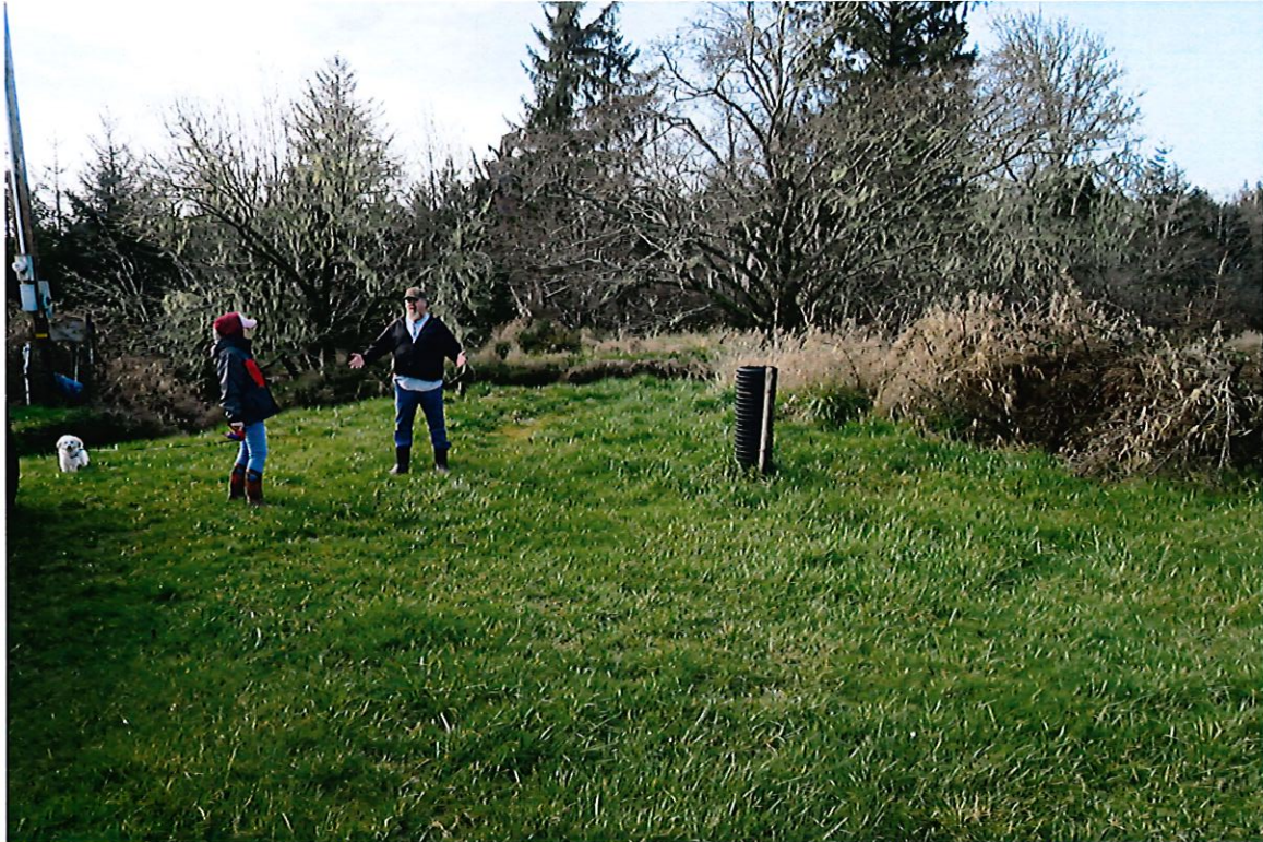
Pipe sticking up protecting meter at Two Mile Creek, electrical meter visible on the left.
