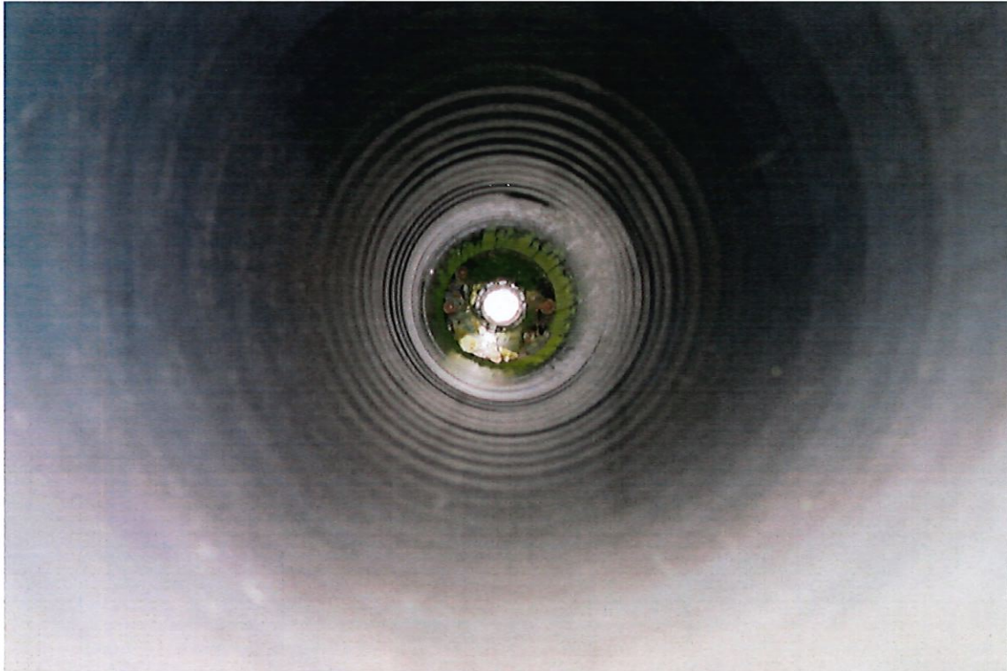
McCrometer totalizing meter, at bottom of pipe, protection from high winter water and silt.
