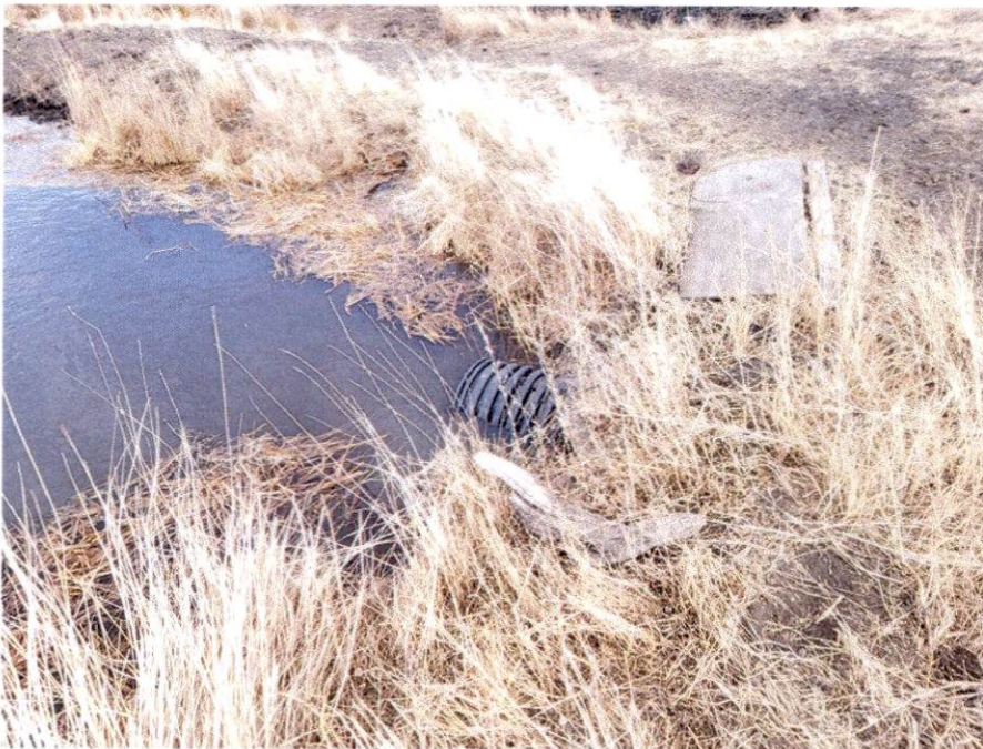
Flooding Distribution Headgates
