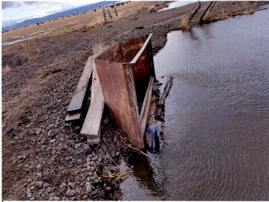
Flooding Distribution Headgate
