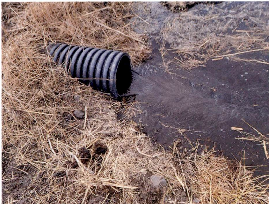
Flooding Distribution Pipe
