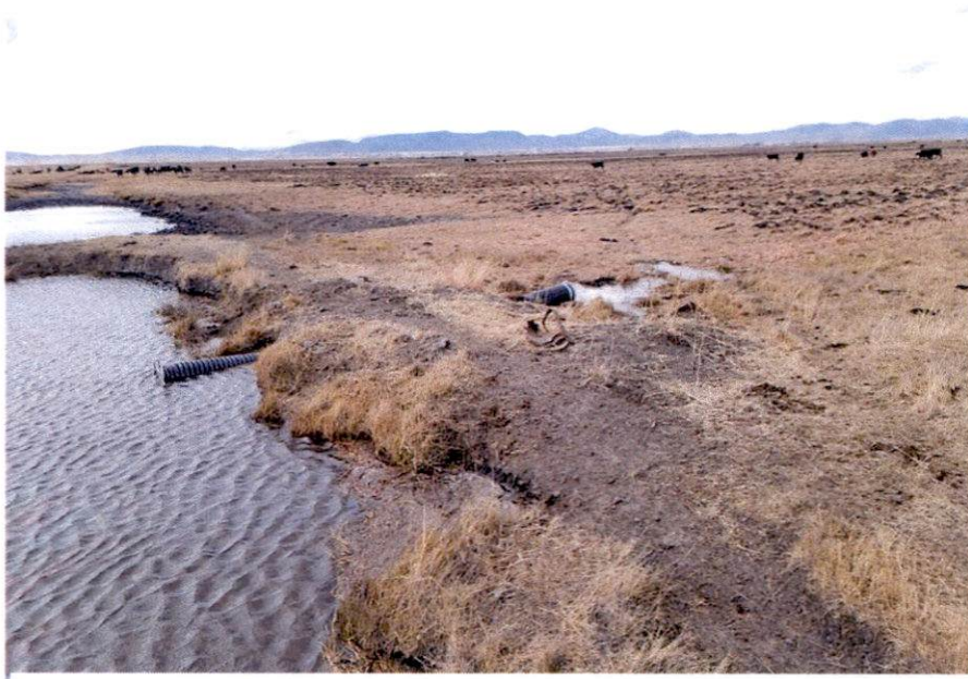
Flooding Distribution Headgates
