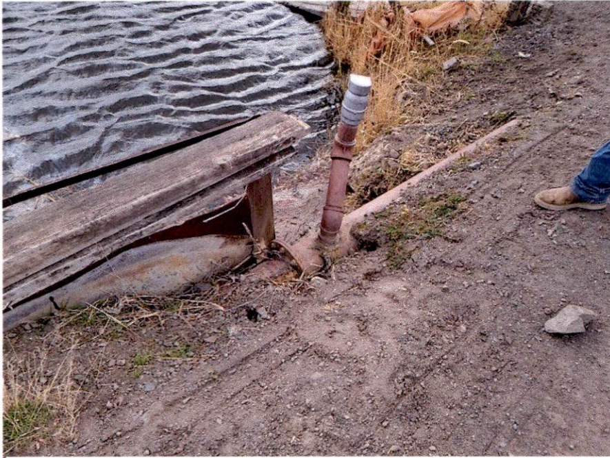
Well #1 Flooding Mainline
