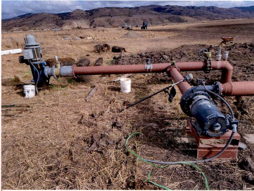
Well #1 & Booster Pump
