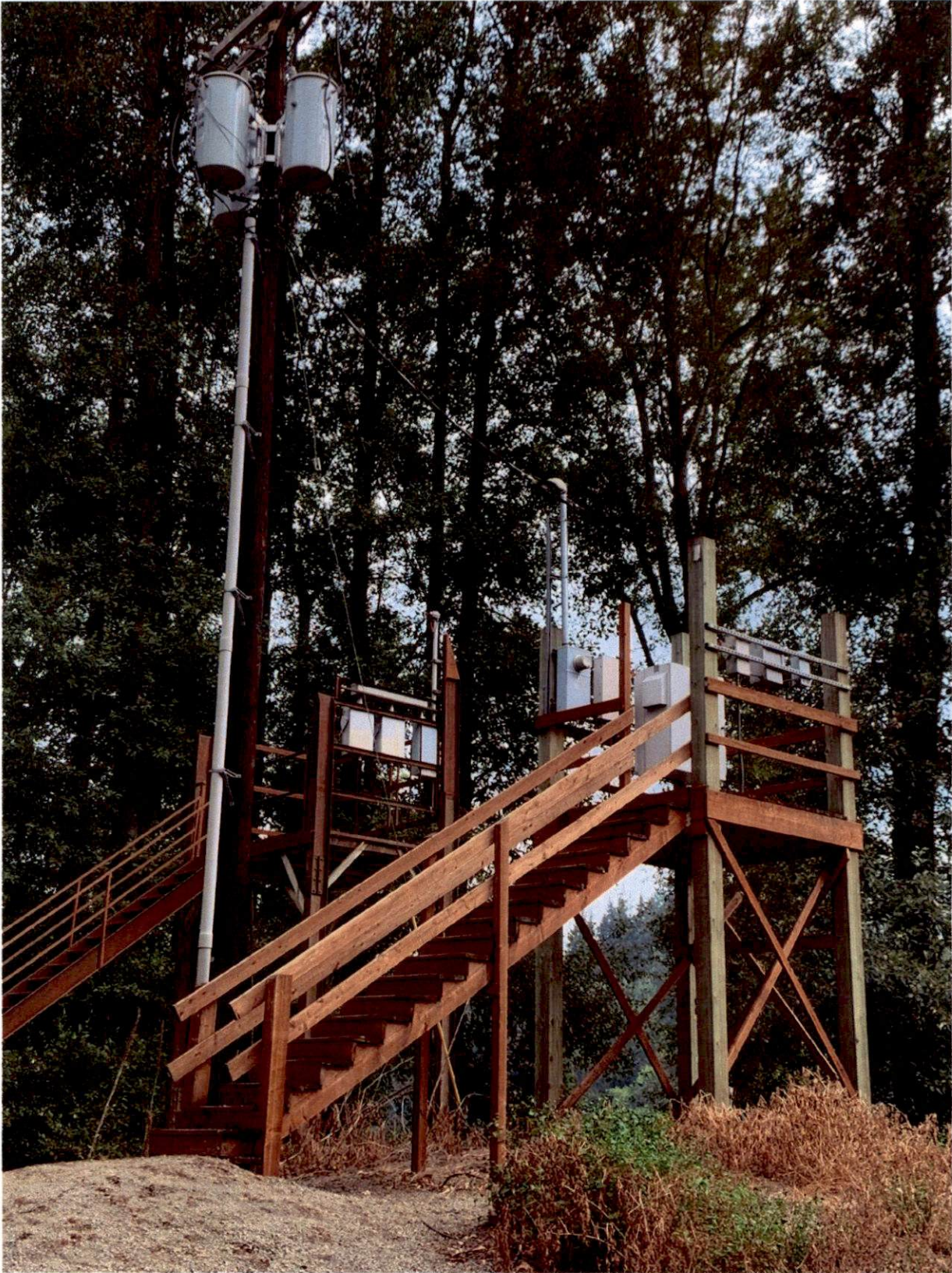
Pump Power Supply and Electrical Panel
