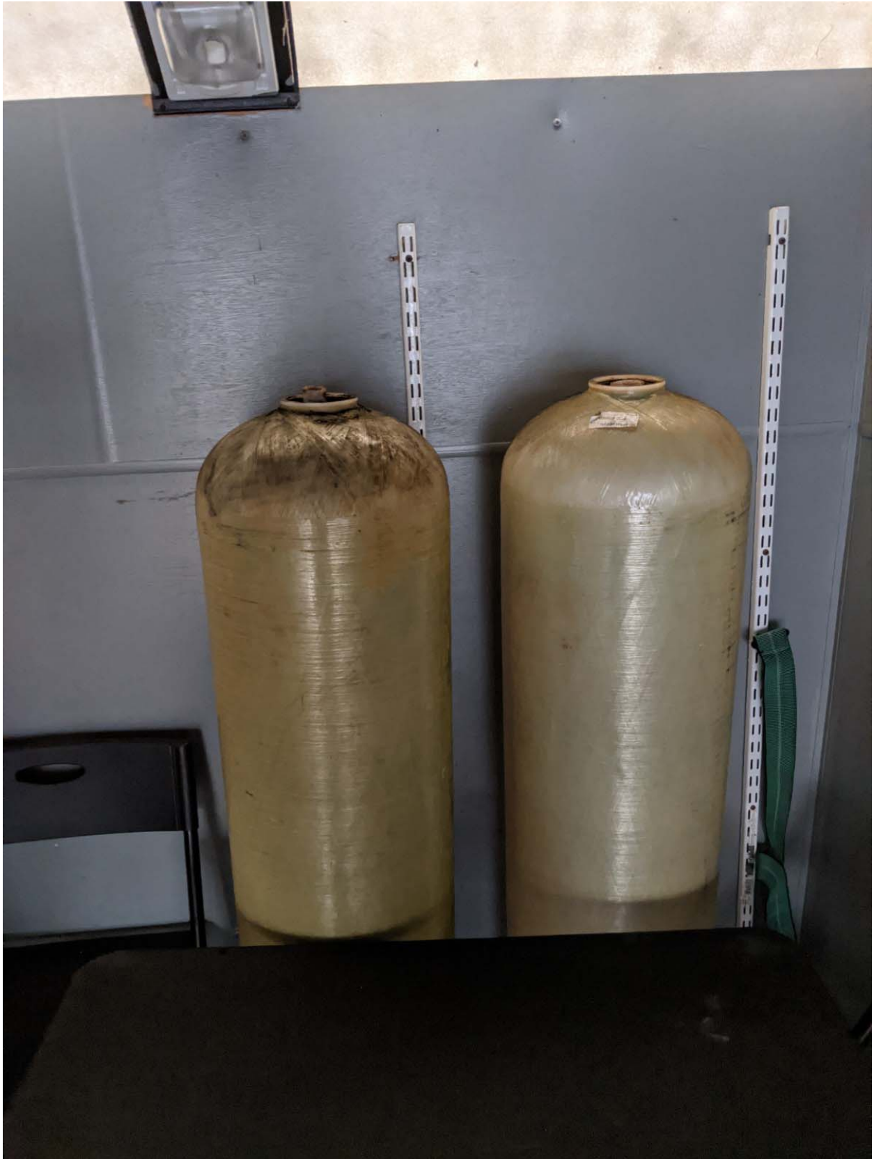
Figure 4. GAC vessels, treatment trains 1 and 2
