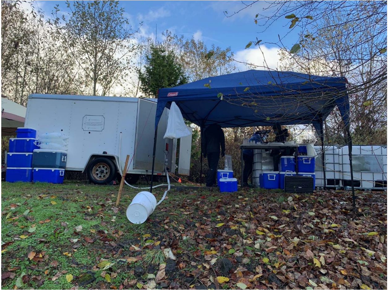
Figure 1. Photo of site setup, with water totes on the right, and the trailer housing the sand filters and GAC vessels on the left.
