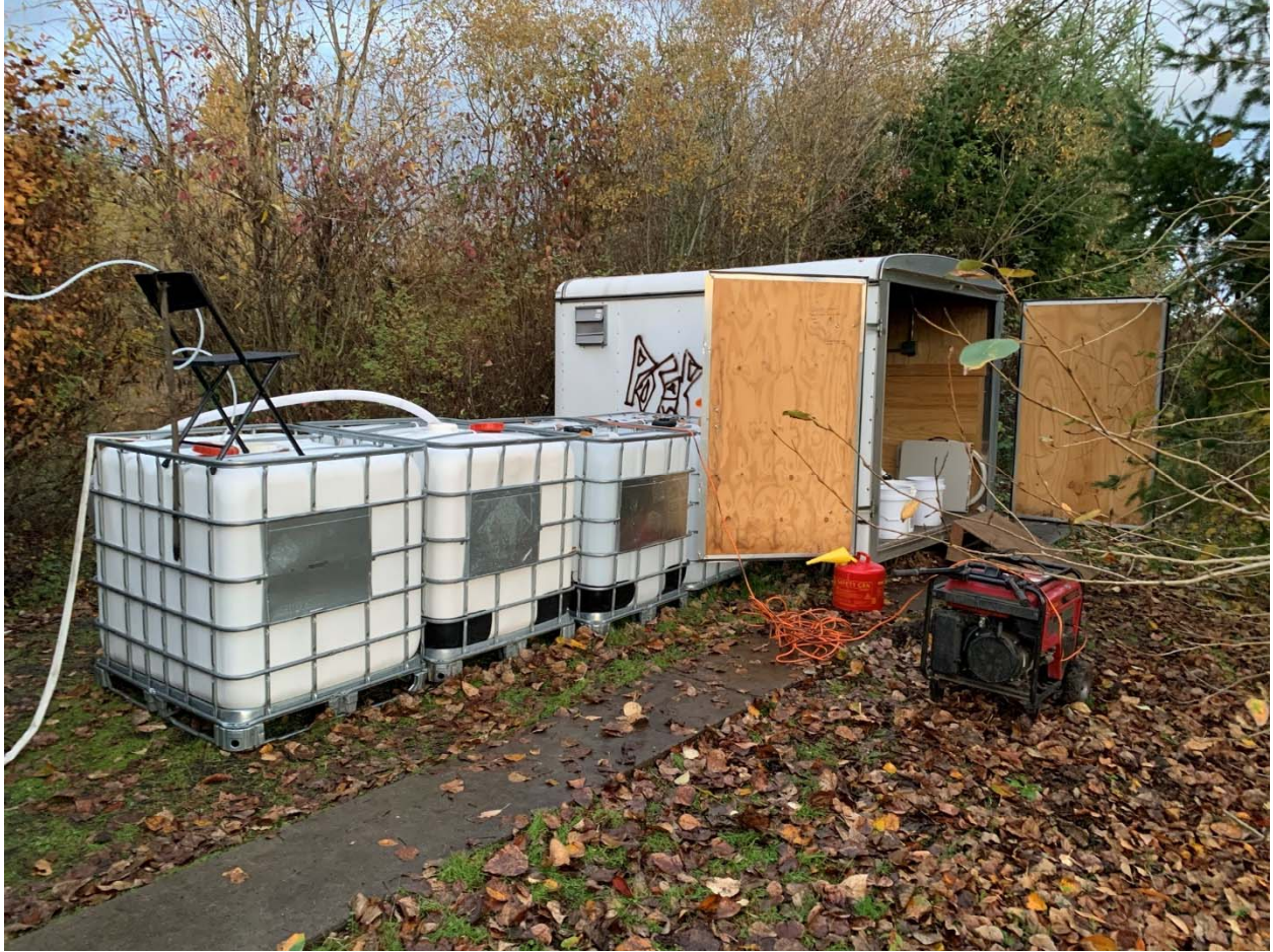
Figure 2. Totes for storing water (left) and the connex box housing the StormwaterRx Aquip and UV disinfection system
