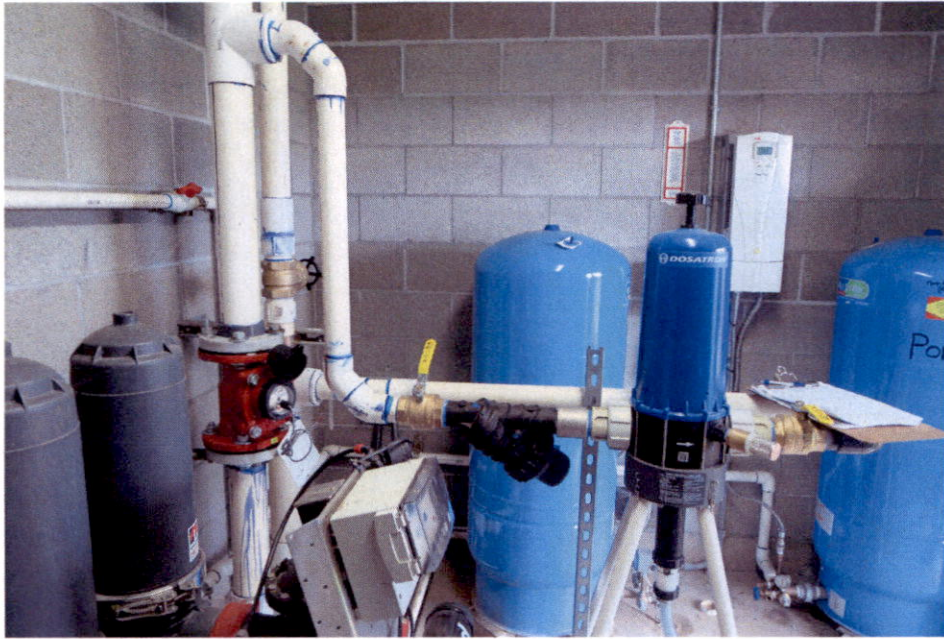
Inside of pump house with meter, controller, pressure tanks and filters.
