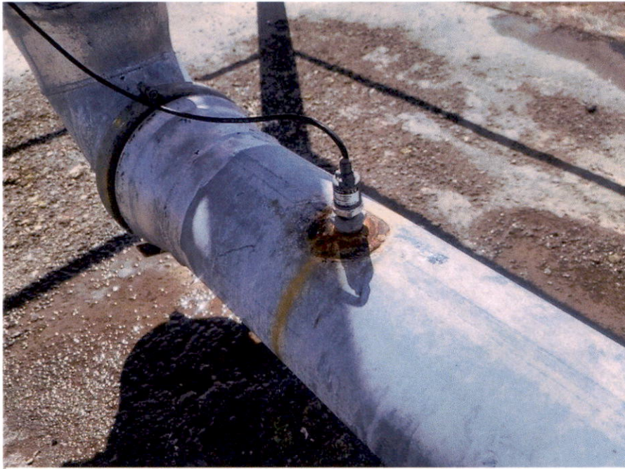
Well #8 Pivot Pressure Transducer
