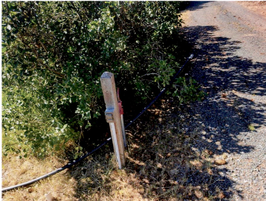
Frost Free Hydrant & Piping for Distribution to Place of Use
