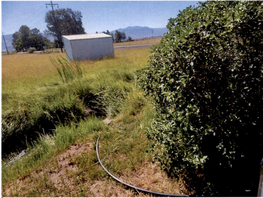
Piping to Place of Use
