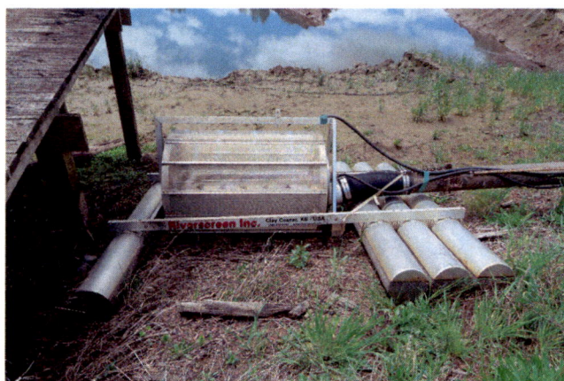
Riverscreen, Active Fish screen in Unger Pond, pond maintenance is underway.
