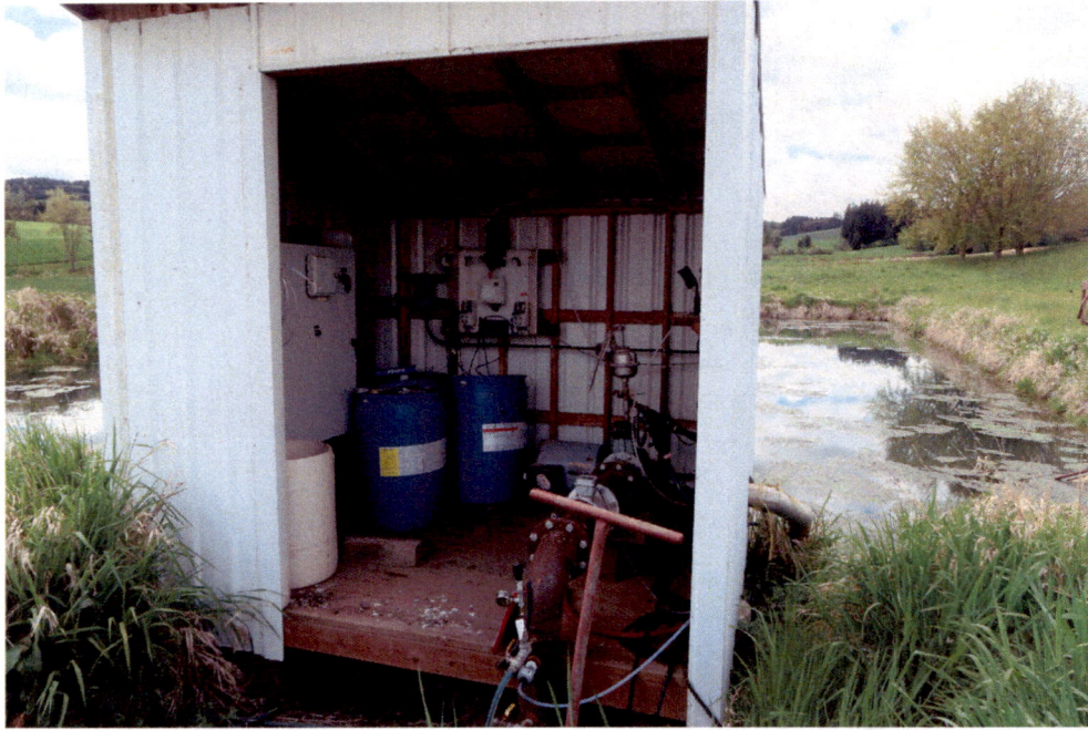
Pump house at sump (bulge) below Grandpa's Pond, pump, motor and meter in shed.
