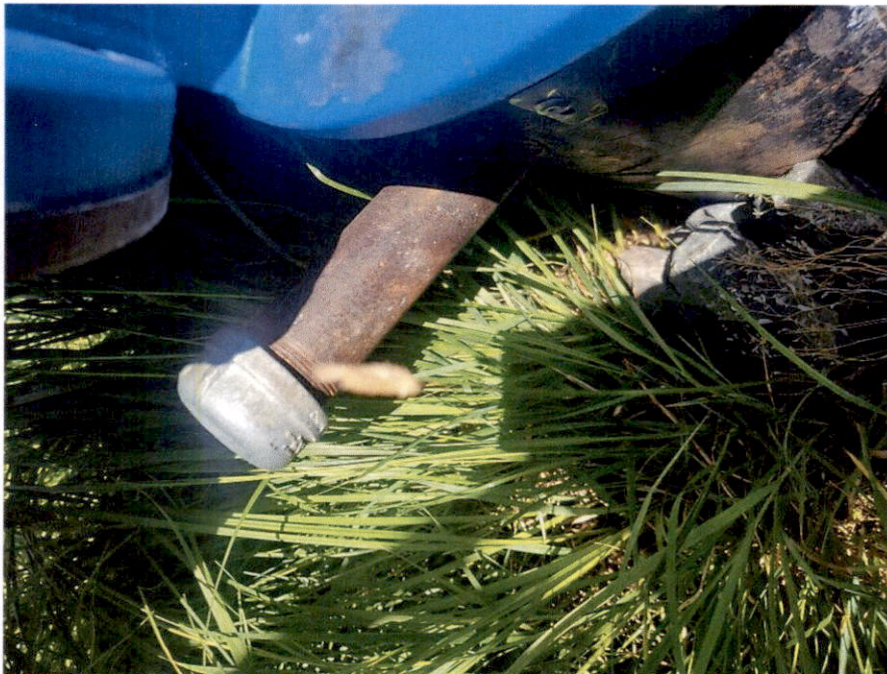
Well #1 Access Port
