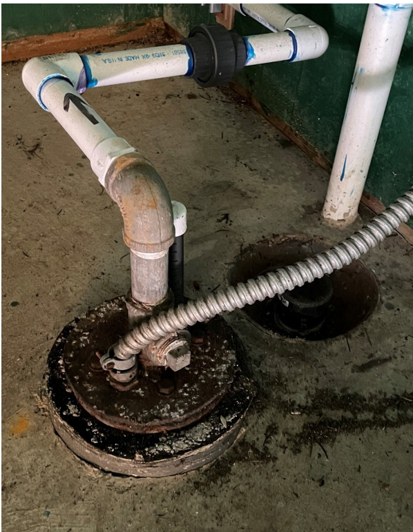
Damaged well, NW Region
