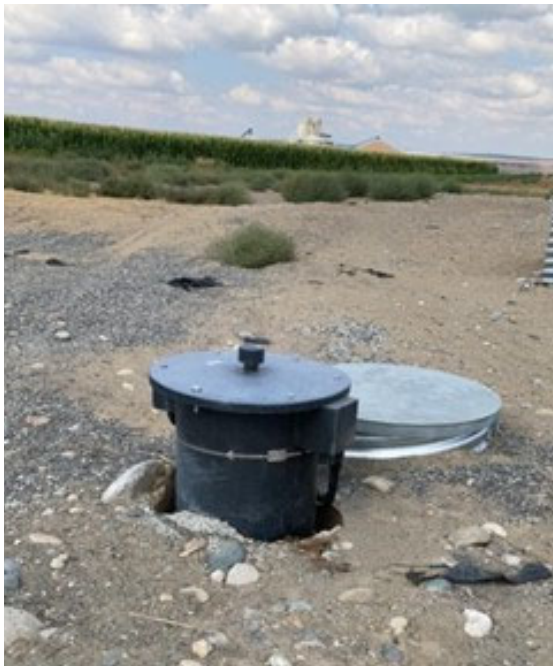
Well with deficient seal in NC Region
