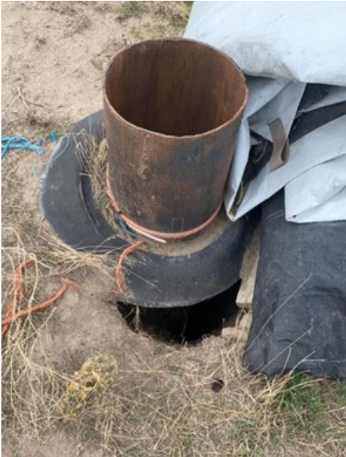
A deficient well seal in eastern Oregon.
