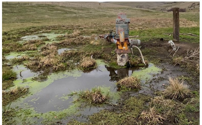
Leaking flowing artesian well in NC Oregon
