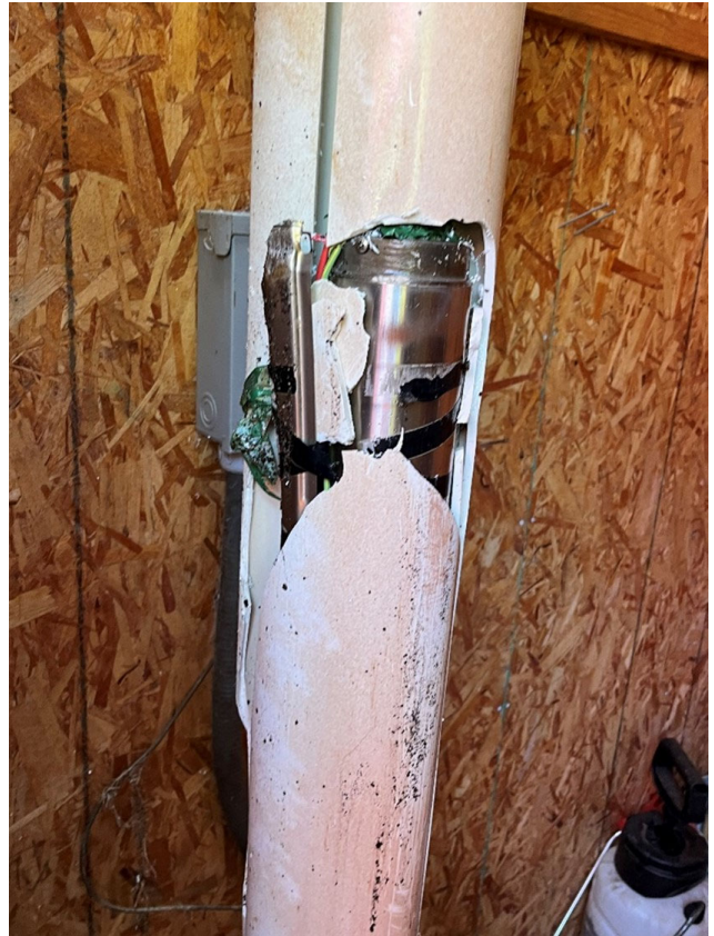
Collapsed liner with a stuck pump
