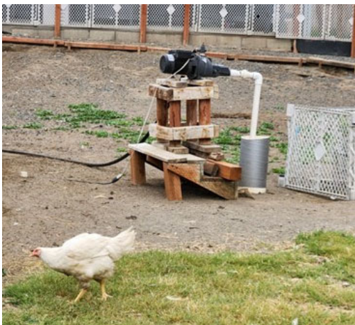
Well constructed by landowner without a permit.
