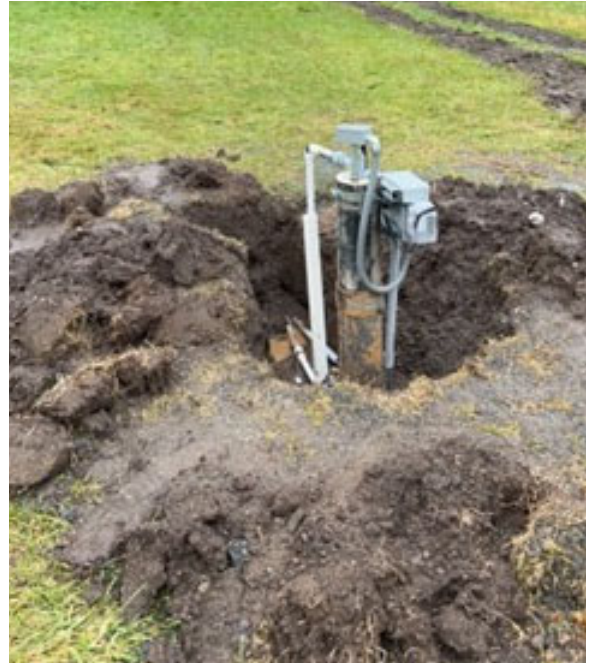
New well with a deficient seal in SW Oregon.
