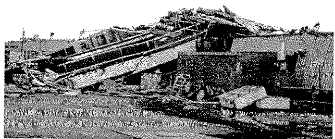
In 1964, the control tower at Anchorage, Alaska International Airport fell during the M9.2 earthquake. It was a split-level structure that was seven stories high on one side and built of reinforced concrete. Photo: USGS
