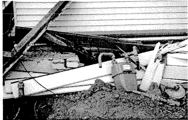
Houses don't need to collapse to be evacuated. This house shifted off its foundation in the 1989 Loma Prieta, California quake and now all the utilities are disconnected. Photo: H. G. Wilshire, USGS
