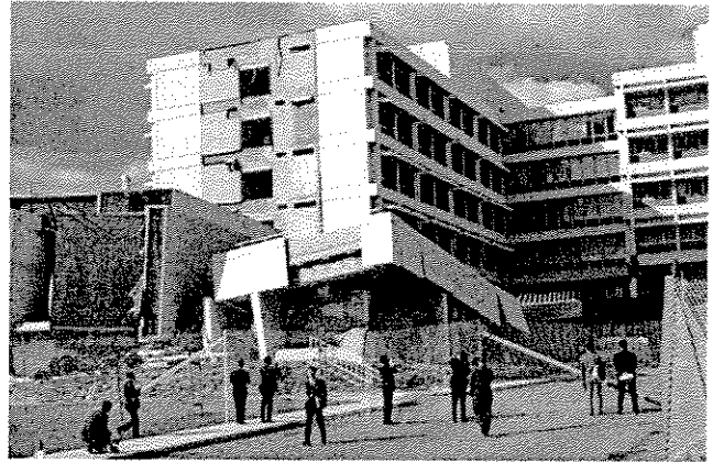
In the 1971 San Fernando, earthquake, the south stair tower (above) fell, and there was other structural damage at Olive View Hospital. Three people died and the building was evacuated. It is imperative to have hospitals and other essential facilities available during the crisis of a subduction zone earthquake. Photo: R. Kachadoorian, USGS
