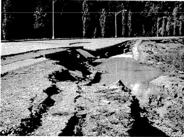
Liquefaction can destroy roads, as the 2001 Nisqually, Washington earthquake did to this street outside Olympia. Many stretches of Highway 101 and other coastal roads in Cascadia are vulnerable to this type of destruction. Photo: T. Walsh, Washington Division of Geology and Earth Resources
