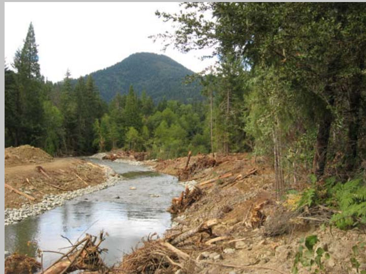
POST-PROJECT: Downstream view immediately after channel construction. Channel includes habitat features and large wood complexes.
