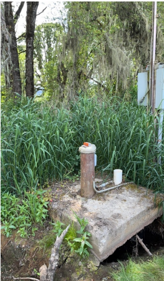
Water well with a deficient seal
