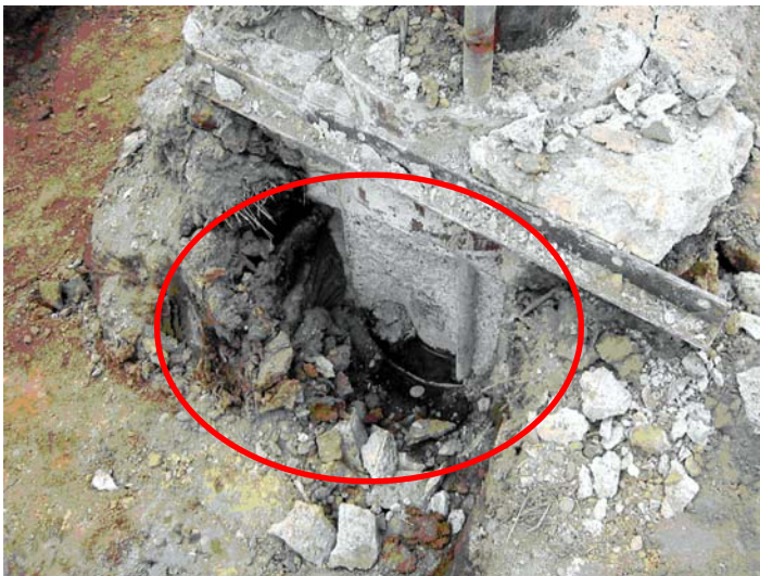
Figure 13. Surface casing left in ground and void in seal.
