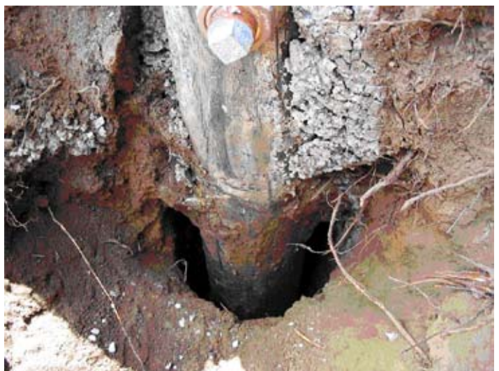
Figure 11. Large void found in well seal.
