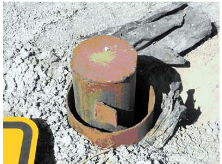
Figure 5. Surface casing left in ground and no seal.
