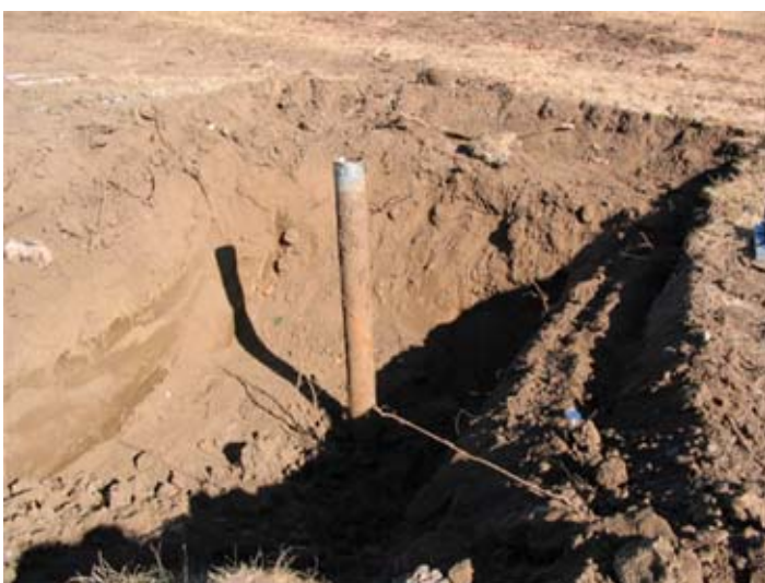
Figure 14. Damaged well at construction site.
