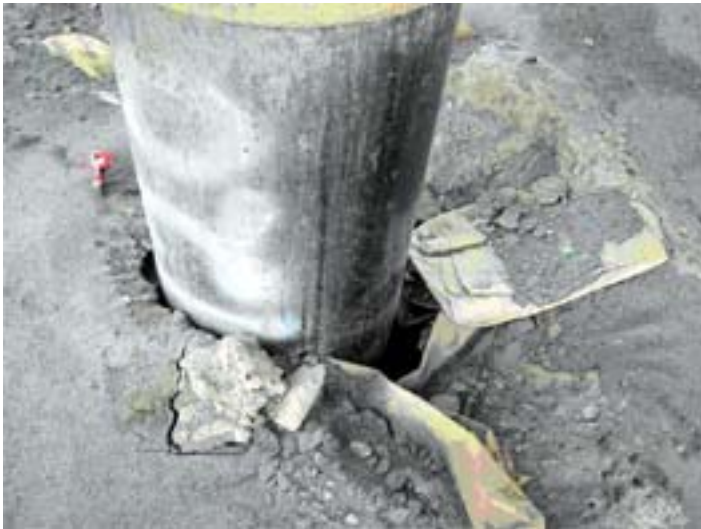
Figure 2. Cement bag seal?
