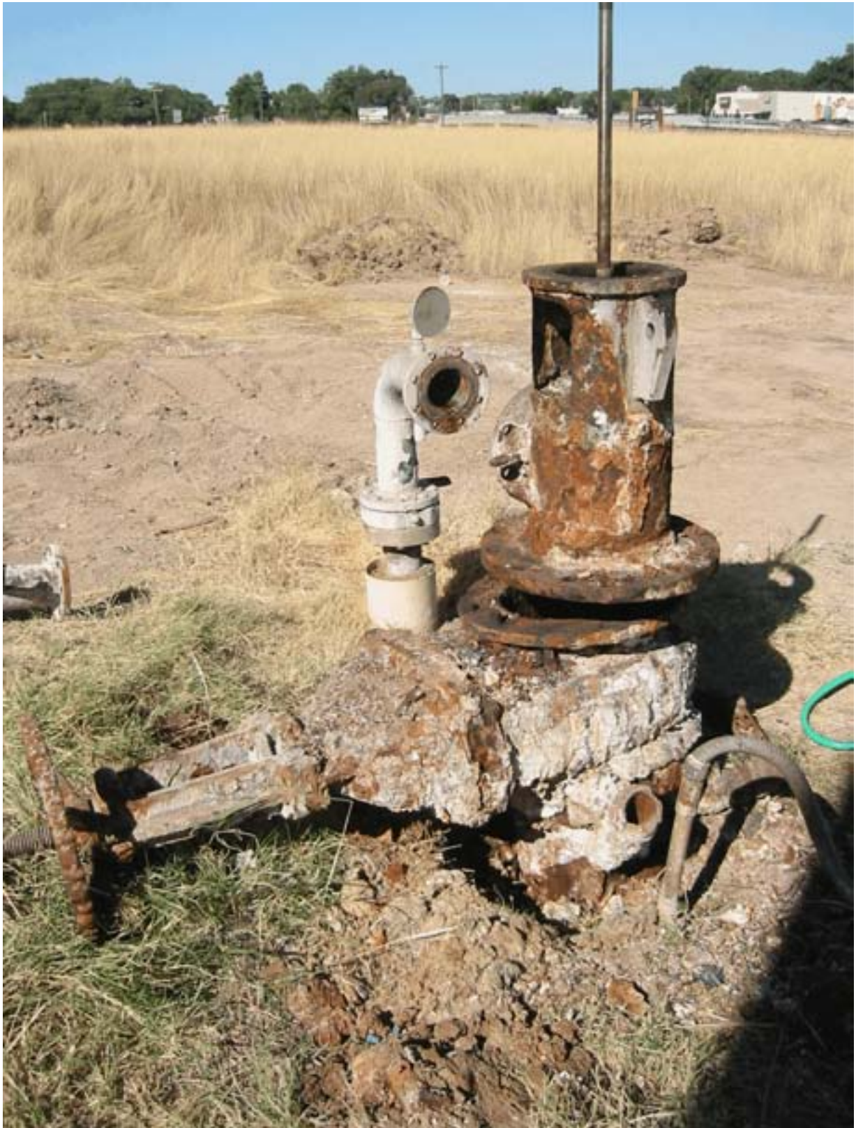
Casing and fittings destroyed by corrosive environment.
