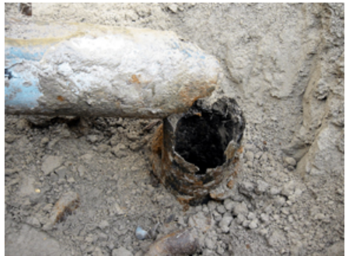
Figure 2. Casing completely rusted through.
