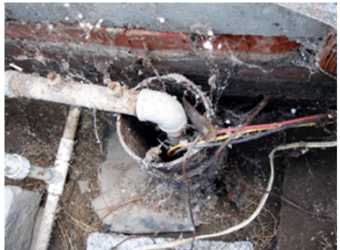
Figure 3. Uncapped cased well in an underground vault.
