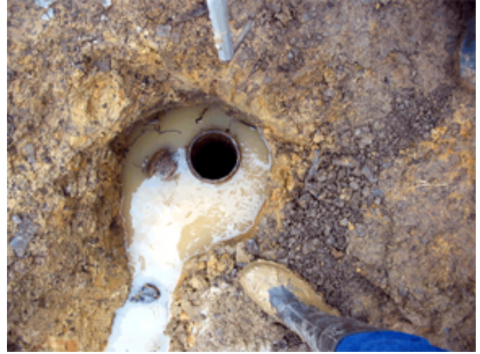
Figure 1. This is a cased well on a construction site. The well head has been cut several feet below grade. Note the water flowing toward the well head. Figure 1B shows debris that was in the well.
