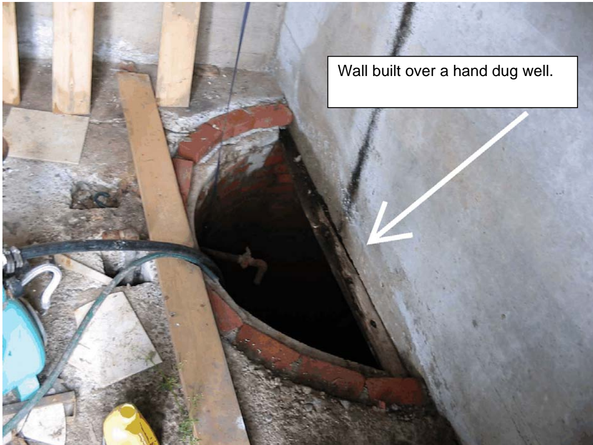
Damaged well hit by excavator.
