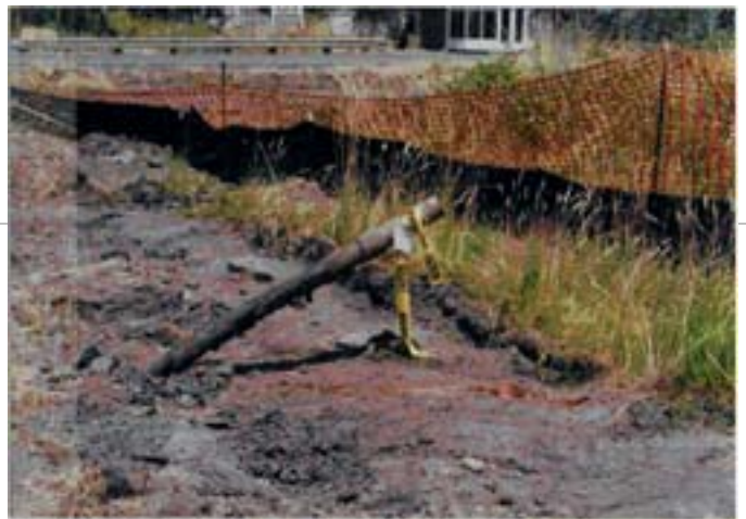
Figure 3. Damaged Water Supply Well.
