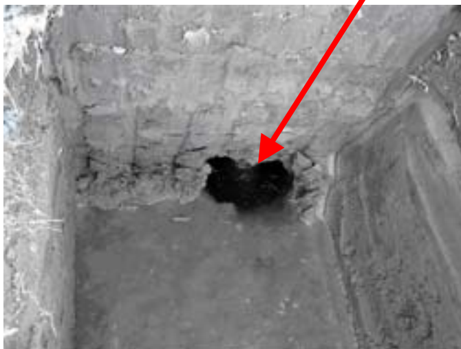
Figure 1. Void in well seal.
