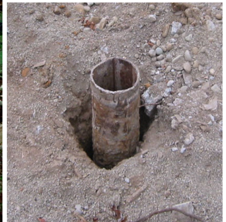
Figure 3: Domestic water well where the seal has disappeared.
