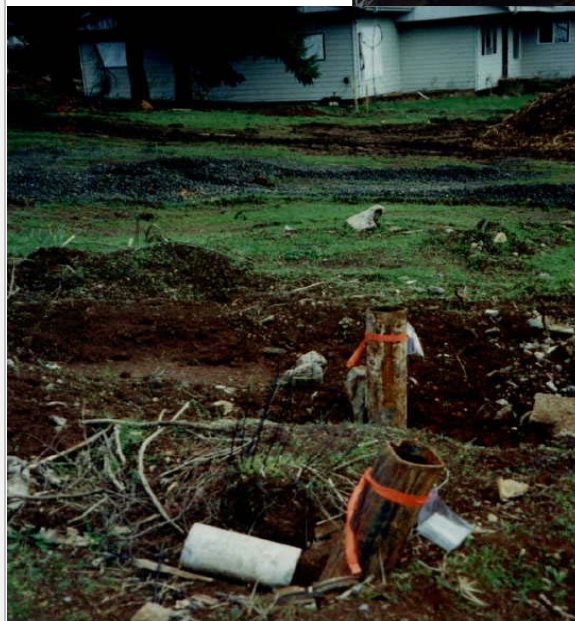
Figure 4: Two water wells damaged by an excavator on a construction site.
