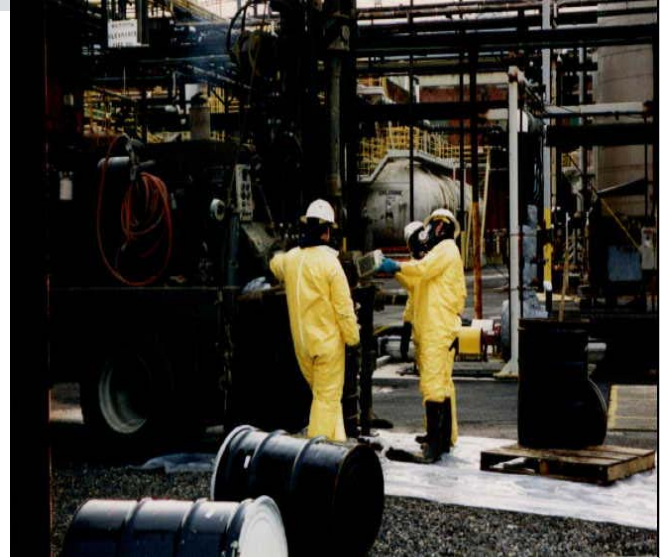
Figure 2: A monitor well being constructed on a contaminated site in Portland, Oregon.
