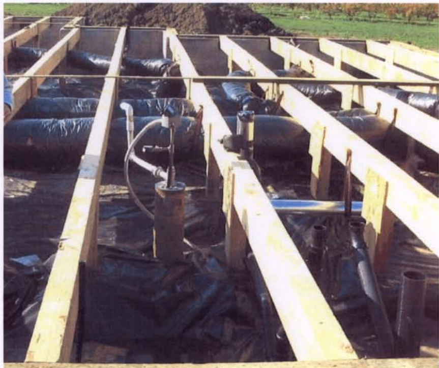
House being built on top of a well. The owner abandoned this well.
