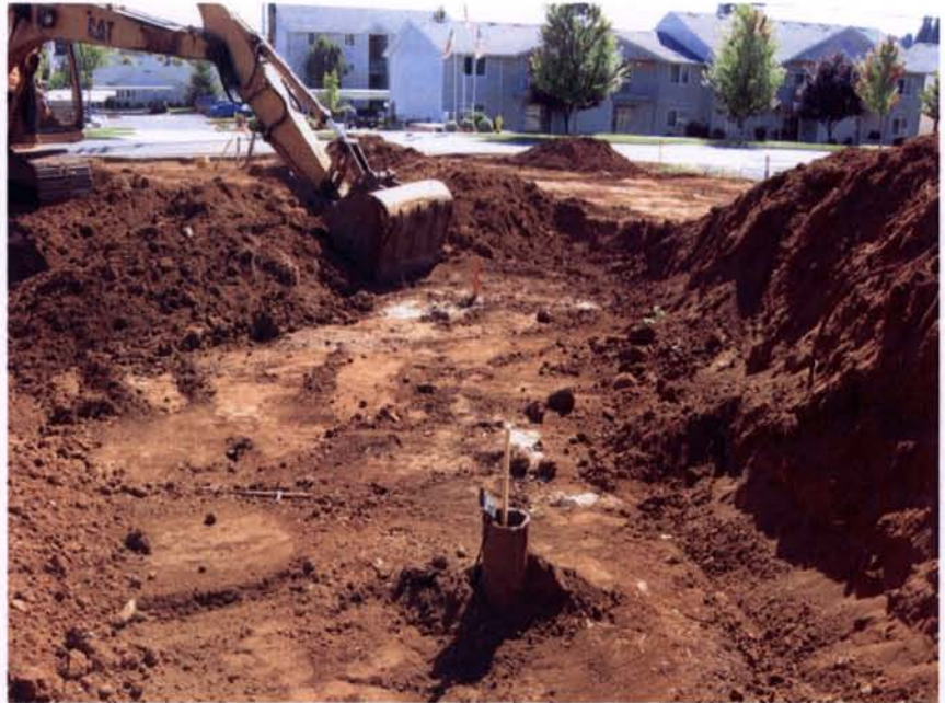
Damaged and buried well at a construction site. The landowner uncovered the well and abandoned it to standards.
