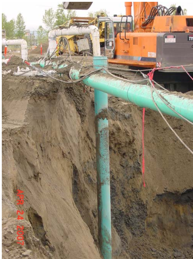
This is a dewatering well that was installed too close to the excavation work. This well has since been abandoned.
