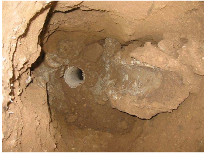
This 2"-inch monitoring well had been broken and buried below land surface. This is what it looked like when it was ultimately located.
