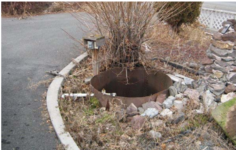
Dangerous Old Dug Well
