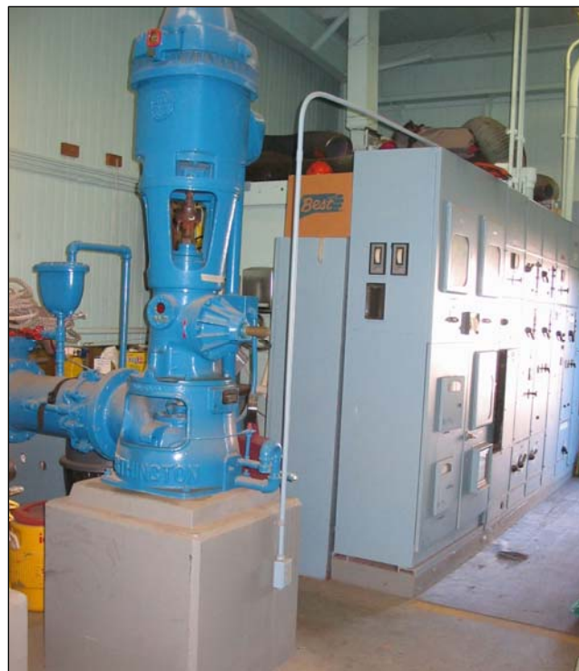
Turbine Pump Pedestal
