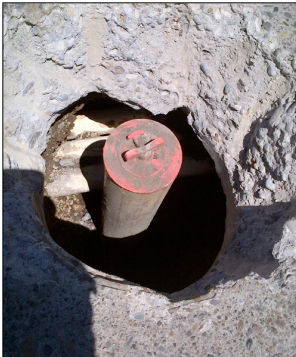
Monitoring Well with buried underground lines right next to it.
