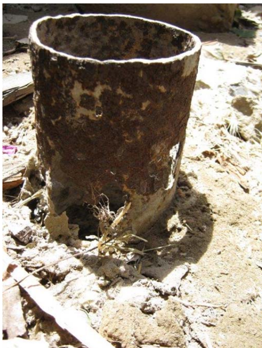
This well casing had significant rust damage, resulting in large holes which allowed access to the aquifer.
