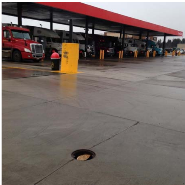
Damaged and uncovered, this monitoring well is directly in the path of large trucks. Without a proper covering, it can easily become a conduit for contamination.
