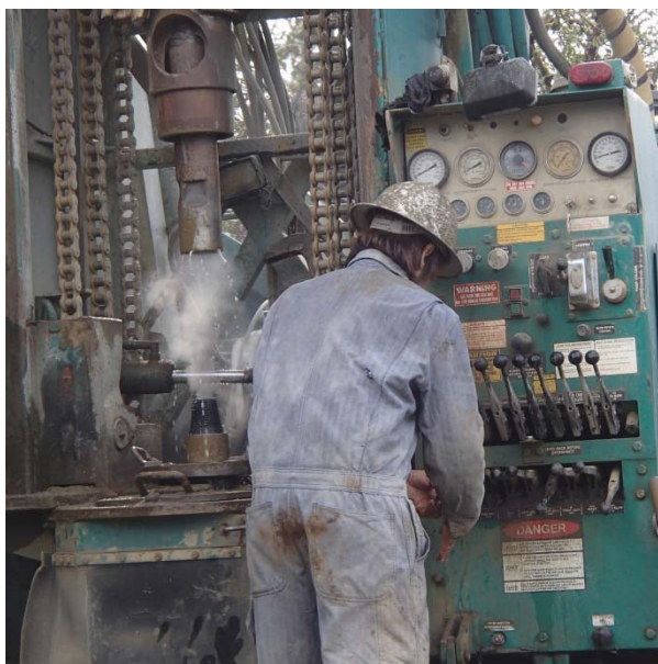
Well constructor working water 'magic'. "Pay no attention to the man behind the... drill rig!"
