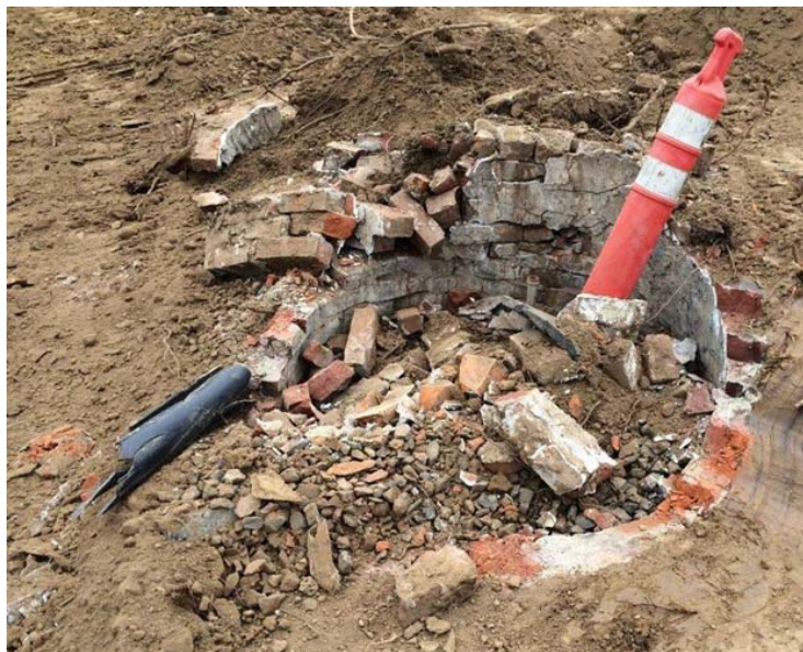
Dug well filled in with debris on construction site.
