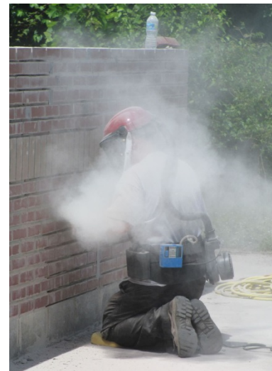
Worker exposed to Silica dust.
