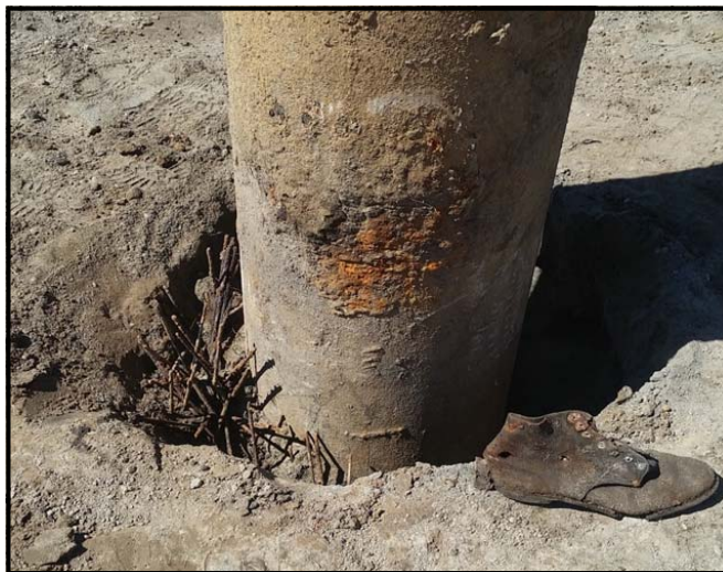
Welding rods and a boot recently discovered in the annular space of an old well being repaired.
