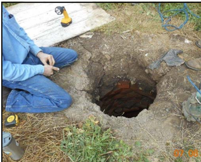
A recently discovered dug well that has since been permanently decommissioned.
