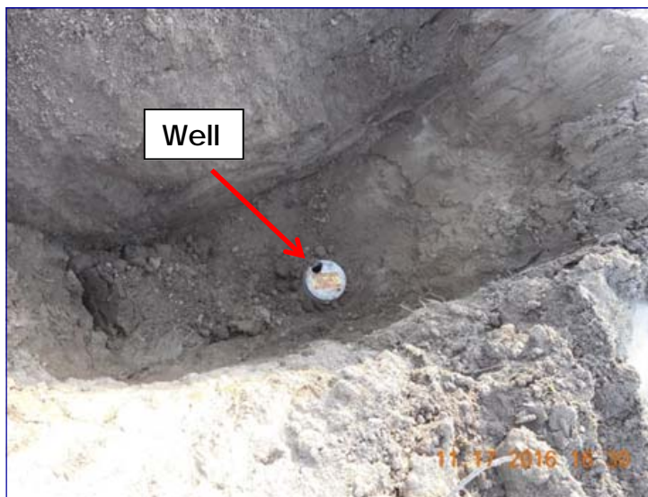
A buried well head with a broken cap.
