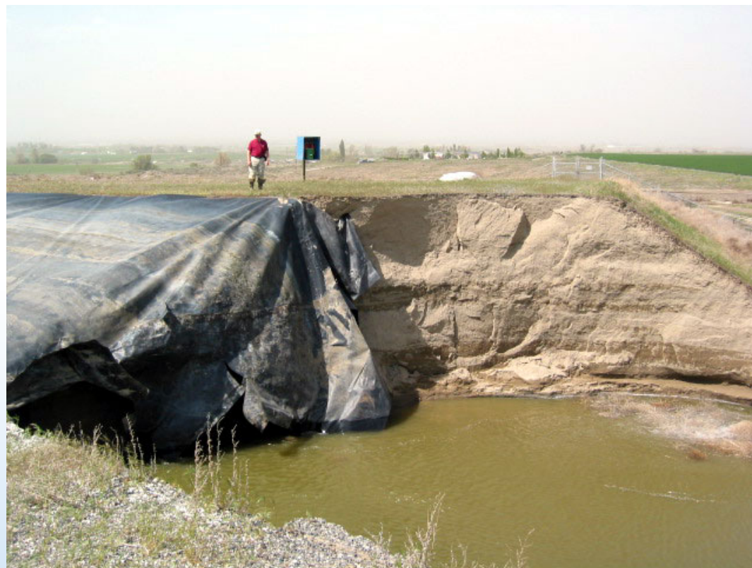
2006 Dam Failure near Hermiston
