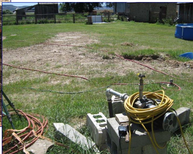
Dug well that is located ten feet from a drainfield.
