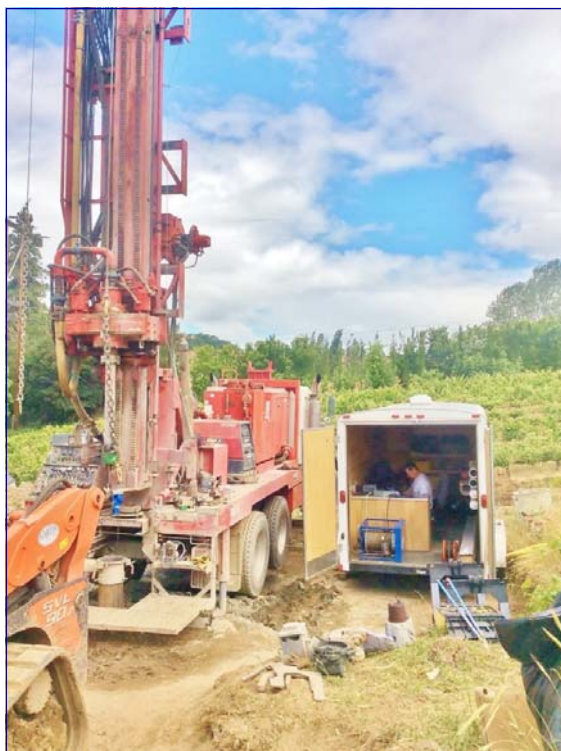
NC Region well inspector using geophysical tools to examine a Mosier area well.
