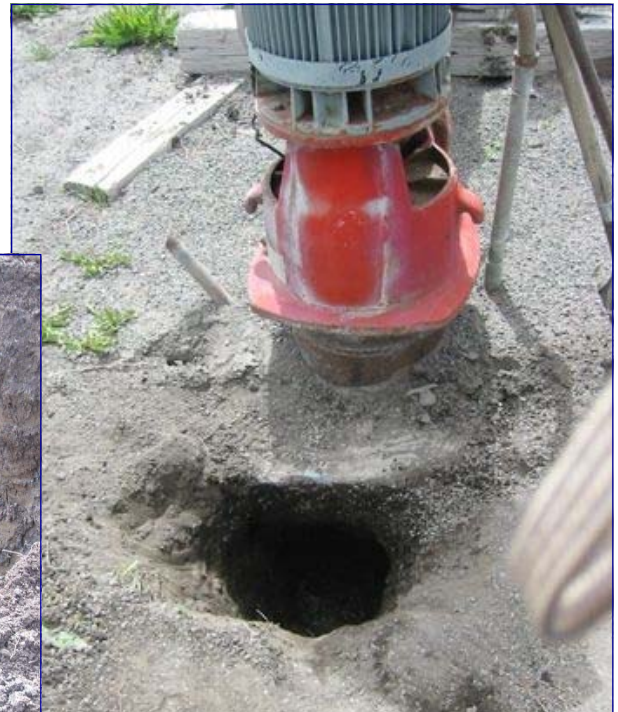
Water well with a bad annular seal.
