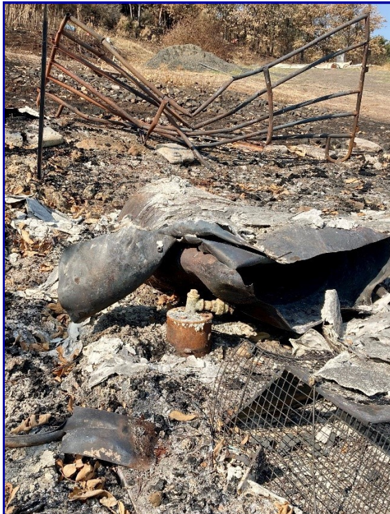
Fire damaged well in SW Oregon
