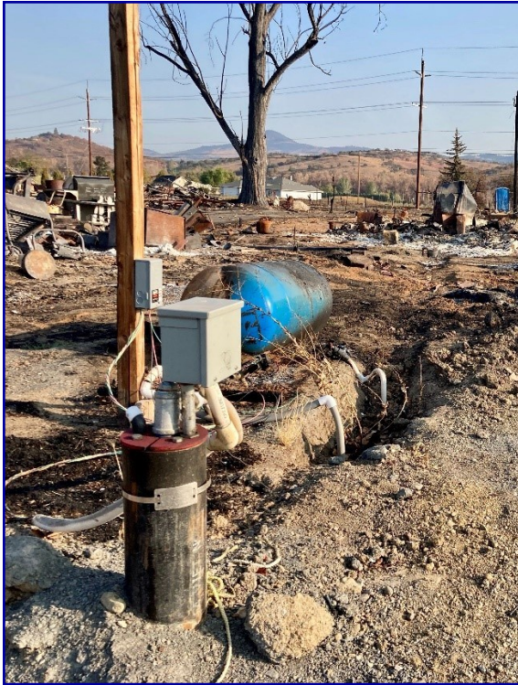
Fire damaged well in Southern Oregon
