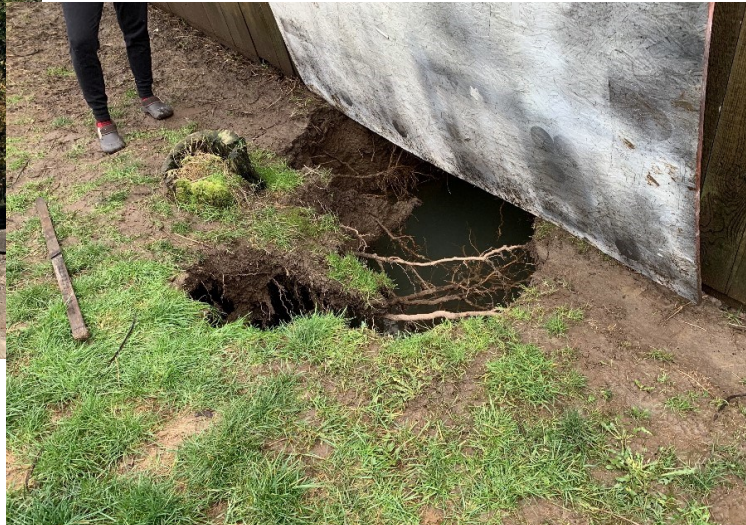
An old dug well that has collapsed.
