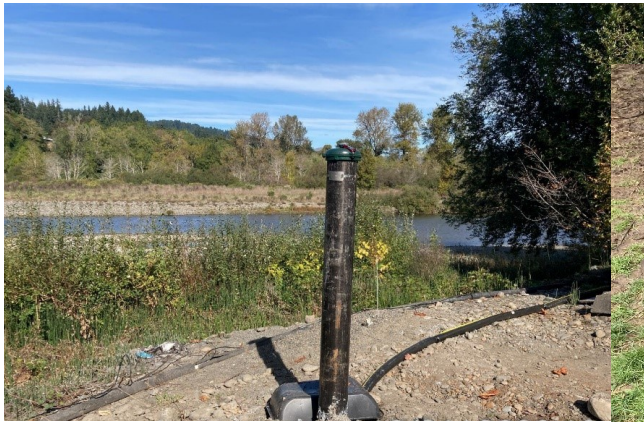
A well that was constructed to allow for seasonal high water level.
