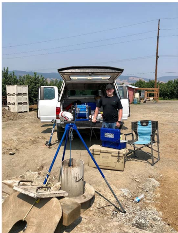
Tommy Laird, NW Region Well Inspector reviewing the construction of a well
